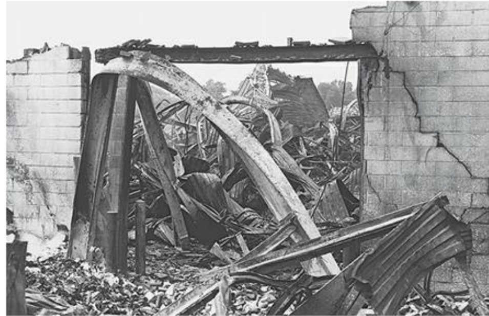
FIGURE 11.66 An exposed steel structure following a prolonged fire in the highly combustible contents of a warehouse.
