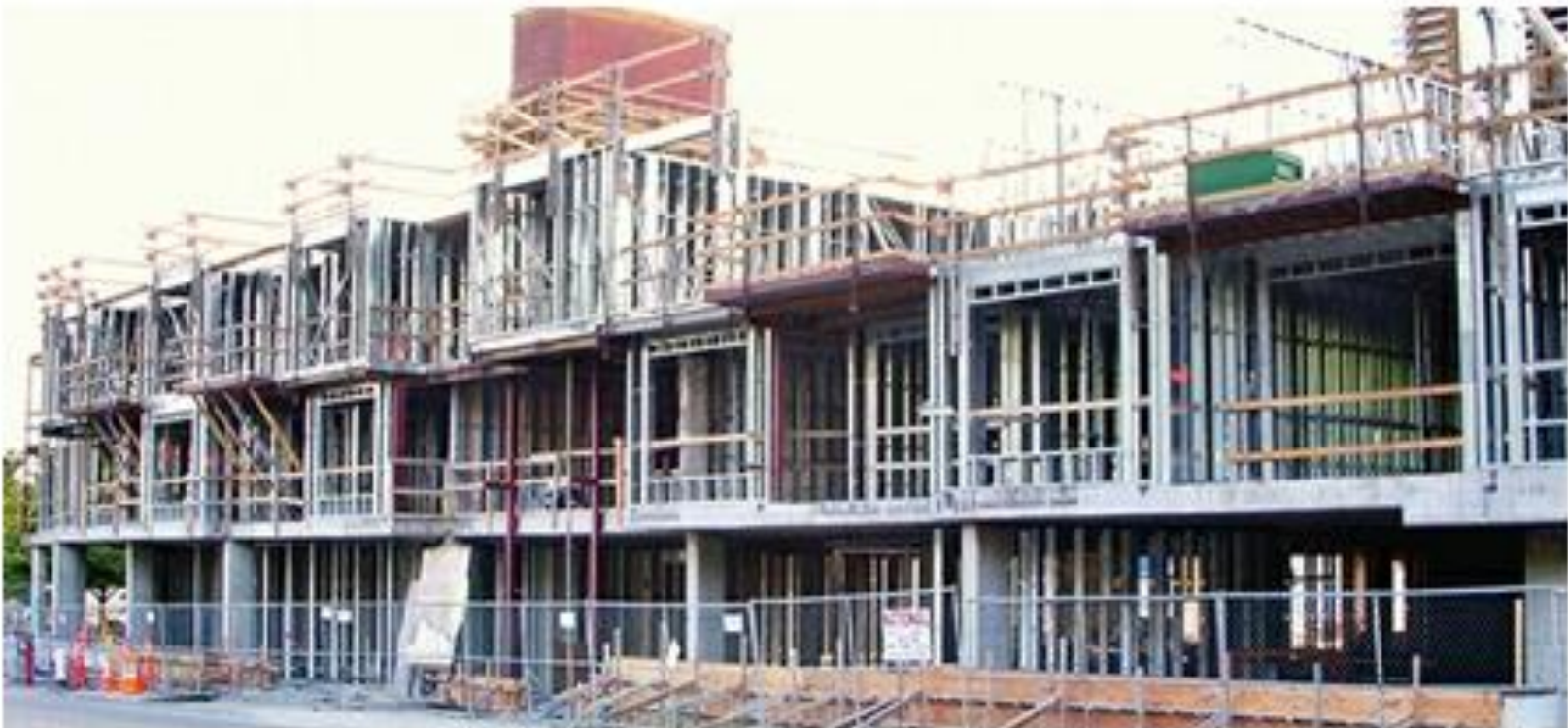
FIGURE 12.18 Light gauge steel stud framing forms the exterior enclosure for this building structured with posttensioned concrete.
