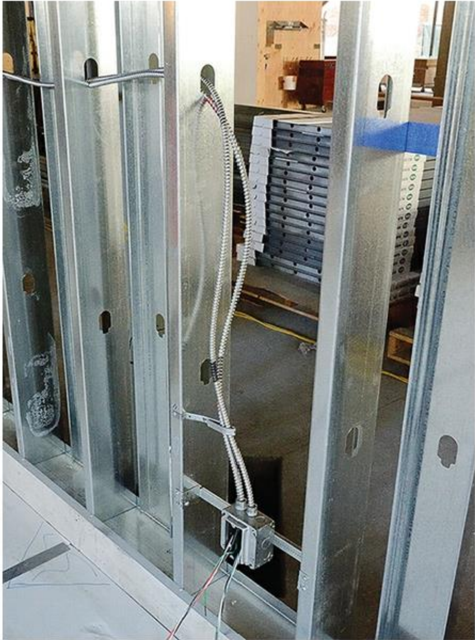
FIGURE 12.11 Flexible metal conduit runs through prepunched openings in metal wall studs. The junction box is supported on metal bracket spanning between studs.
